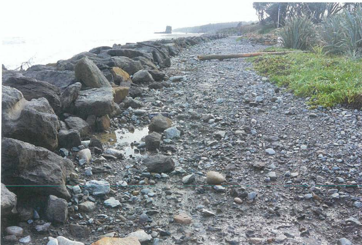
Punakaiki Seawall crest damage.
